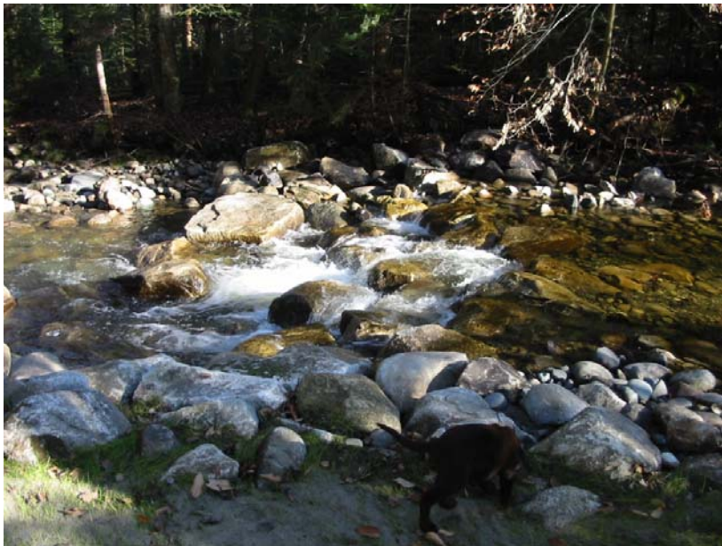
Photograph at the rock weir with fish passage channels from the left bank at Culvert #2 (Middle) taken on November 12, 2010 during moderate flow.
