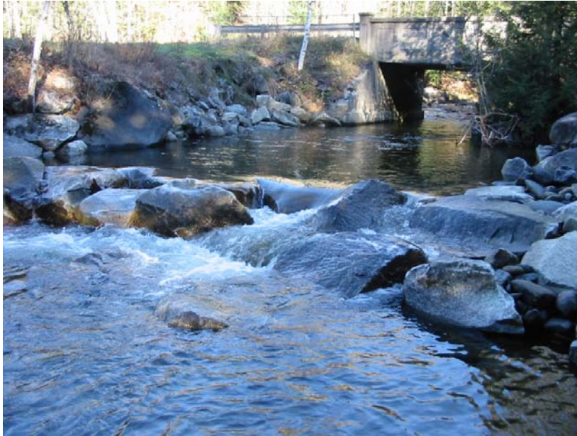
Photograph looking upstream over the rock weir with fish passage channels and backwatered Culvert #3 (Lower) taken on November 12, 2010 during moderate flow.
