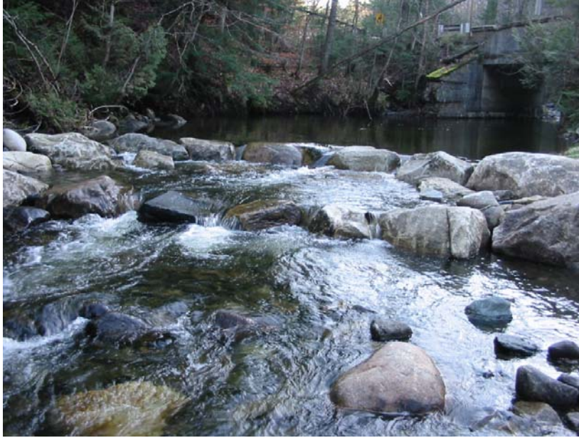
Photograph looking upstream over the rock weir with fish passage channels and the backwatered Culvert #1 (Upper) taken on November 12, 2010 during moderate flow.
