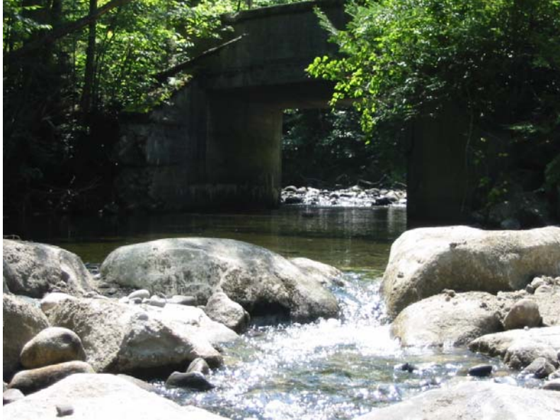
Photograph looking upstream over the rock weir with a fish passage channel and the backwatered Culvert #1 (Upper) taken on August 13, 2010 during low flow.
