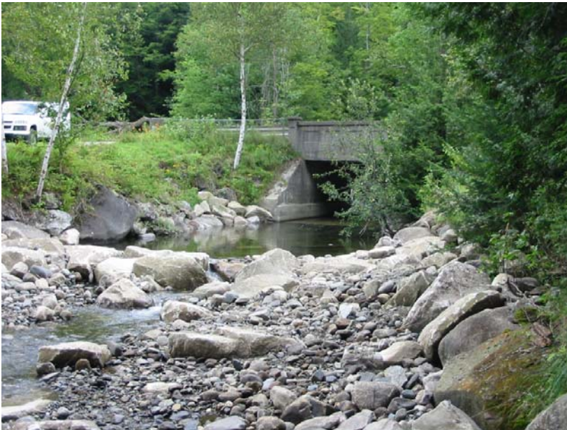
Photograph looking upstream over the rock weir with fish passage channel and backwatered Culvert #3 (Lower) taken on August 13, 2010 during low flow.
