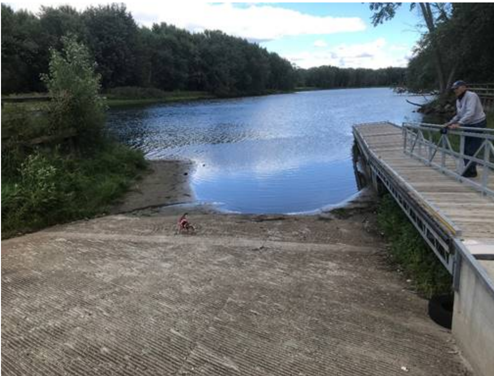
Figure 4. Severe siltation issues on the Colchester Point Fishing Access Area ramp on the Winooski River in Colchester Point.
