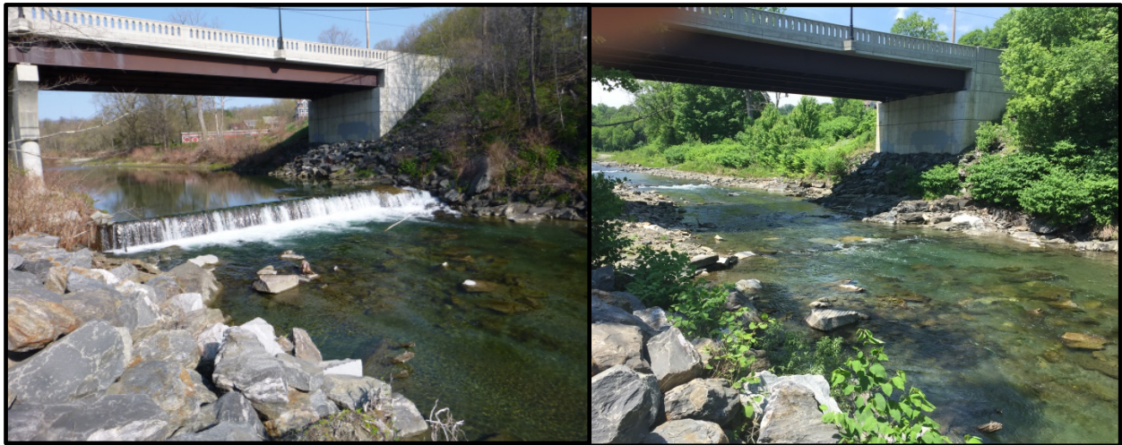
Figure 6. Pre and post photos of the Sargeant Osgood Roundy Dam removal in Randolph, VT. Project partners include American Rivers, TNC, White River Partnership, VDEC and VFWD.
