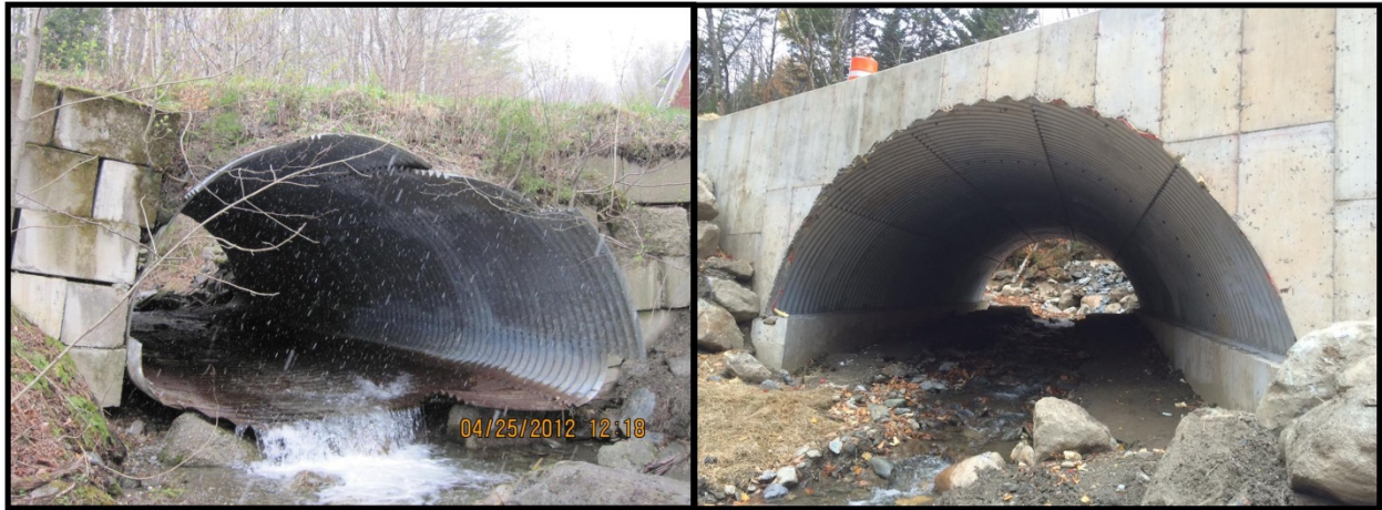
Figure 5. Pre and post culvert replacement photos from Bradley Brook in Warren, VT. Project partners include the Friends of the Mad River, USFWS, USFS, Town of Warren, Winooski Natural Resource Conservation District and VFWD.
