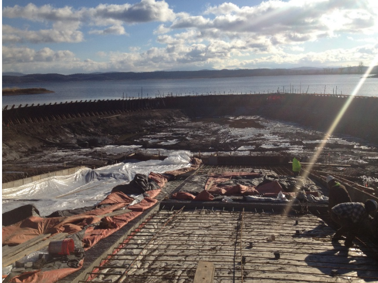
Facing east, looking at a port-a-dam used to dewater Lake Champlain in order to dredge the lake bottom and install the double land boat ramp.
