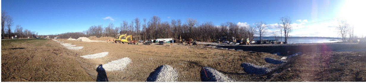
Figure 1. Panoramic view of the active construction of the John Guilmette Fishing Access Area parking lot. December 2014 looking north from US Rt 2 in Milton.
