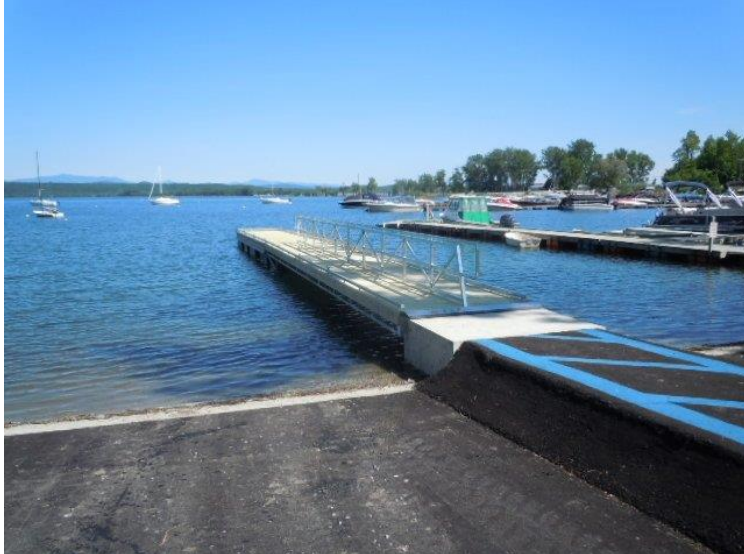
Similar view as the above photo after the port-a-dam had been removed and the ramp installed along with the 70 ft ADA accessible dock and walkway.
