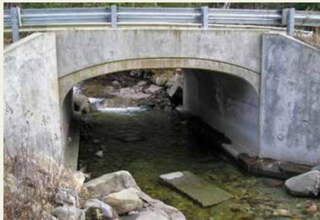
Newly designed culverts provide flood resiliency and allow fish to move freely throughout the stream.
